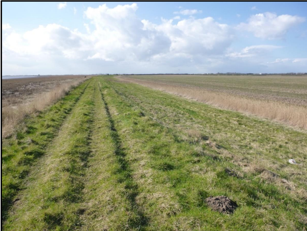
Plate 8.7: Existing embankment, looking west across East 2, with Soak Dike on the right-hand side.
